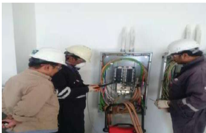
Pre-commissioning of Power Panel
