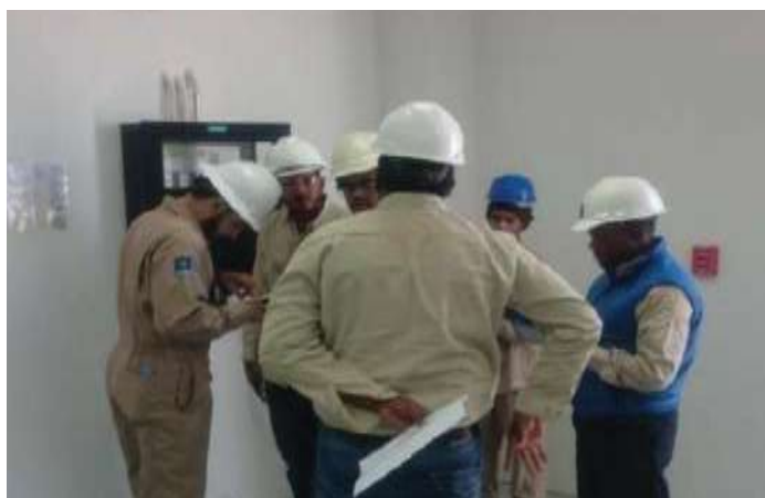
Pre-commissioning of FACP
